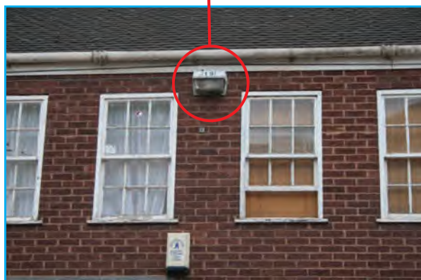
Inconspicuous lighting units on buildings help to minimise clutter in this village high street.
