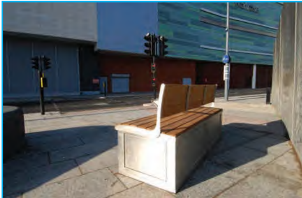
Bench containing traffic signal controller
